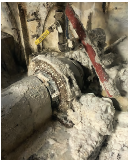
Proper setup and attention can reduce sealing failures in a horizontal pulpers.
