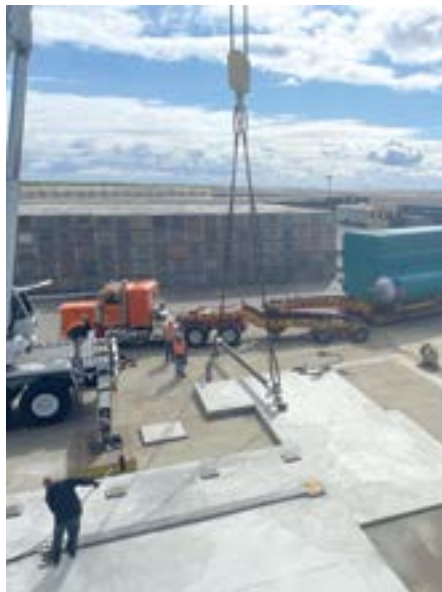
180,000 lb/hr. in stock boiler delivery for expedited replacement project.
