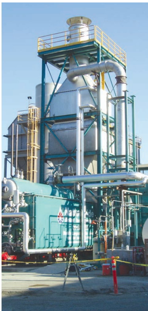
A 120,000 lb/hr package watertube rental boiler with CataStak™ SCR for single-digit NOx compliance.
