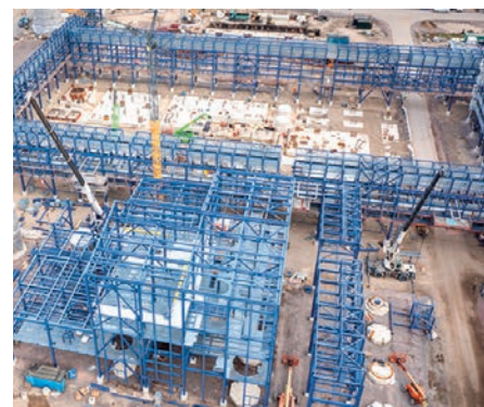
With UPM's expanding biofuel and biochemicals businesses – including, notably, the Leuna biochemicals refinery currently under construction in Germany – operations throughout these process and chemical industries require significantly more strict process safety management.
