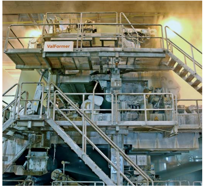
In a rebuild project at Stora Enso Suzhou PM 1, a SymFormer was rebuilt into a ValFormer and SymPress II was rebuilt into a SymPress B shoe press.
