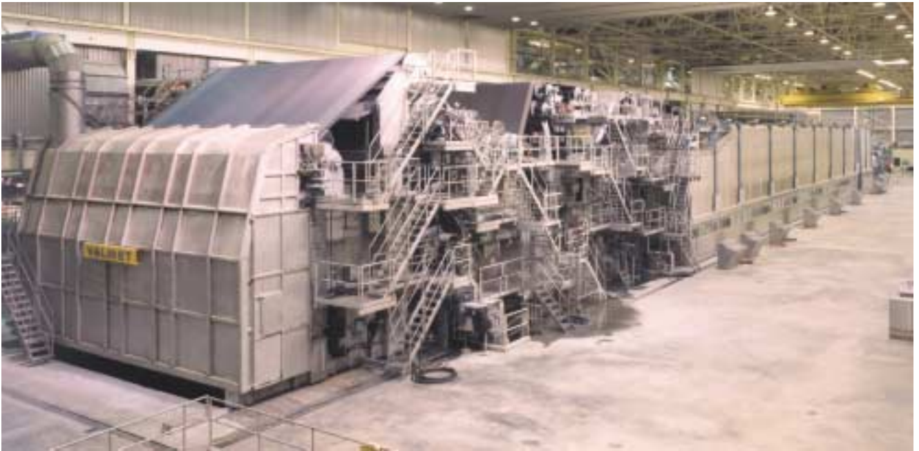
No. 2 PM at Dublin is a Metso (Valmet) SpeedFormer HS that was rebuilt in 1998 to include a shoe press, one of the first such newsprint applications. It has operated at speeds as high as 5,800 fpm so far this year and is well along the road to breaking the world records it set last year.
