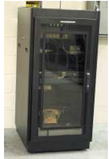
A network communications kiosk was installed on the machine floor to connect each intelligent device to the In.Site Continuous Support service.
