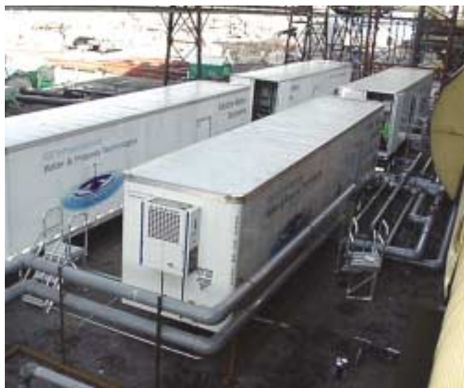
Mobile water treatment trailers in place at a production facility.
