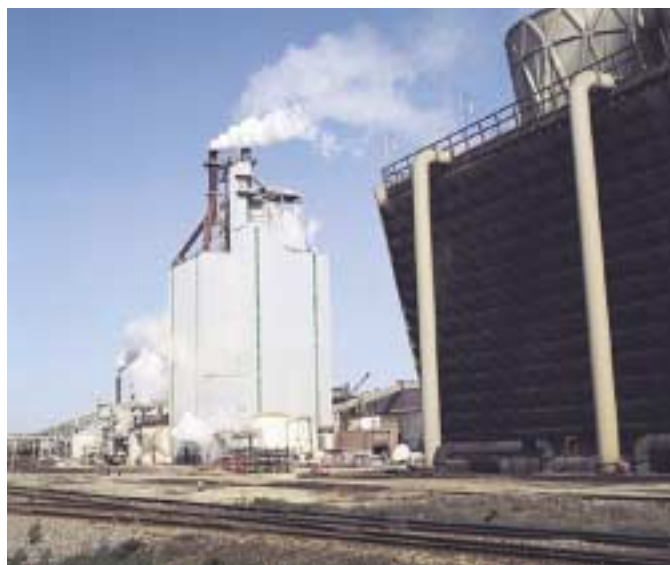
Pulp and paper mill power boiler and water cooling tower (on the right).
