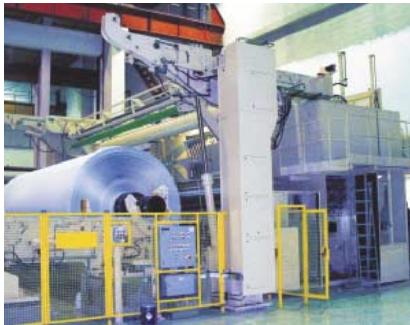
The VariFlex L winder at Ruzomberok operates at maximum speeds of 2,500 m/min and includes storage for parent rolls and reel spools.
