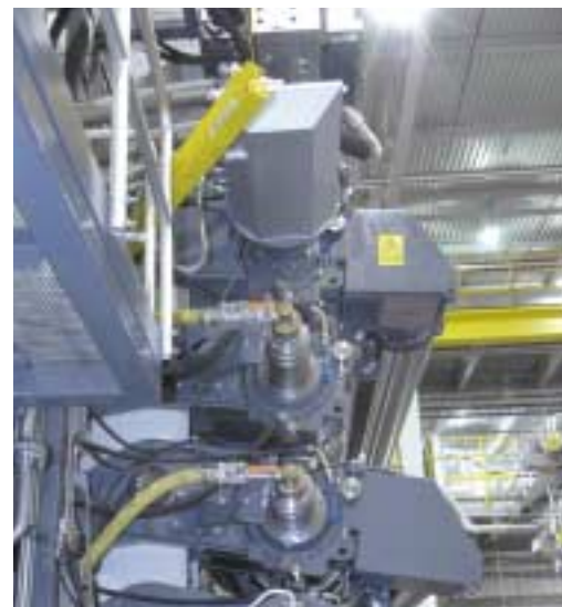
The 8-roll OptiLoad supercalender has three Thermo rolls, two multizone-controlled SymCD/HP rolls on the top and bottom positions, and three polymer rolls.
