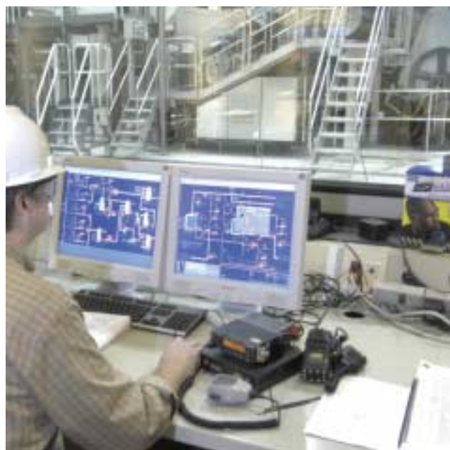
The online OptiCoater, designed for high speed production, uses film coating technology for superior paper surface properties. It is followed by a TurnDry air dryer and two rows of electrical infrared dryers. Coat weight profile of the film transport station is provided by IQCoatWeightCD.
