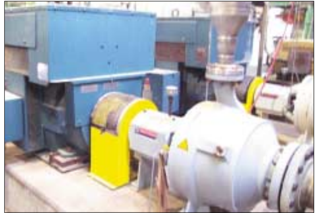
1250 HP, 1200 rpm, 3 phase, 60 hertz, 2300 volts, WP-II enclosed, driving stock pumps.
