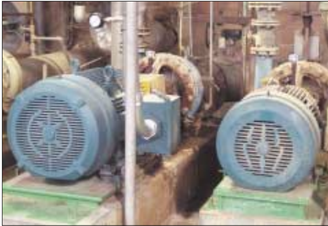
125 HP and a 200 HP, 1800 rpm, 3 phase, 60 hertz, 460 volts, IEEE 841, Reliance driving process water pumps.
