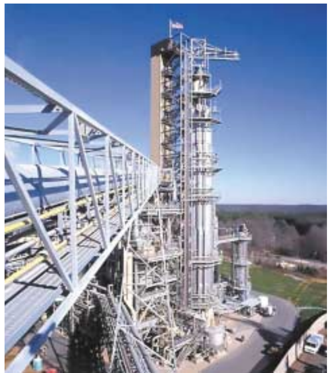
The 225-ft continuous digester, centerpiece of the Catawba's new fiberline, uses low solids cooking for lowest kappa number and highest fiber quality.
