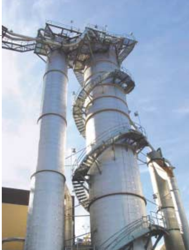
Oxidized white liquor is used in the two-stage oxygen delignification towers, reducing kappa numbers from 30 with the old bleach line to 14 entering the bleach plant.
